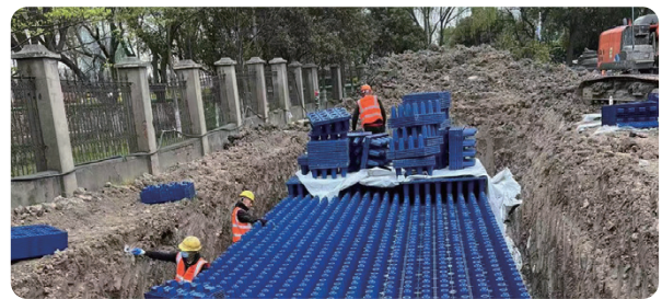
| Taicang CIMC Rainwater Harvesting System |
