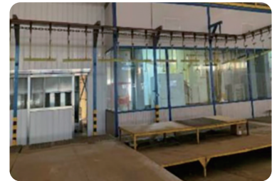
Coating Line with Isolation Installed
